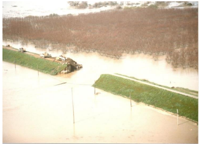
Levee break – rock filling. Marysville Maintenance and Shop 3 are to the left.
